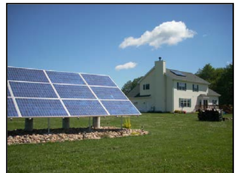
Residential solar array
