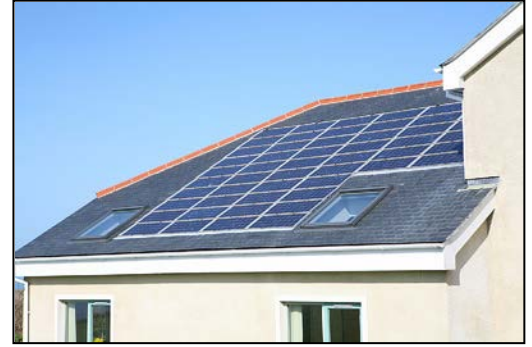
Solar collection system
