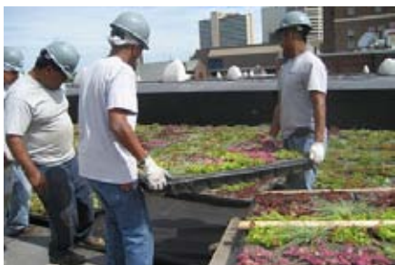
Workers install Hartford's first green roof on the Betty Ruth and Milton B. Hollander Foundation Center. photo: www.commonground.org
