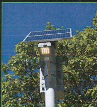
Solar Powered Lighting
