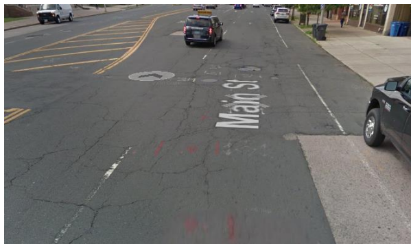
Alligator cracking and potholes on Main St
