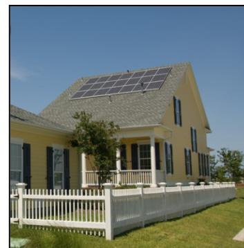
Residential solar panels
