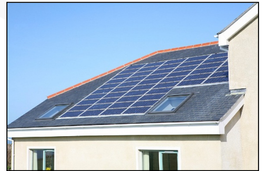
Solar collection system
