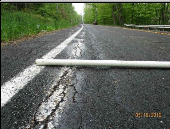
EXISTING: PAVEMENT SURFACE CONDITION
