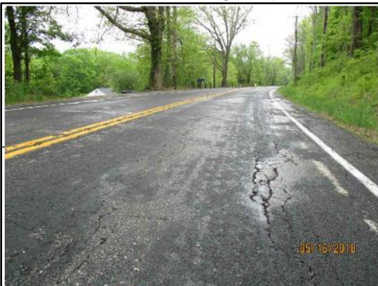
EXISTING: PAVEMENT SURFACE CONDITION
