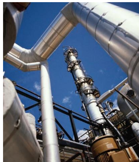
Pipes at an industrial facility. (Source: DHS)
