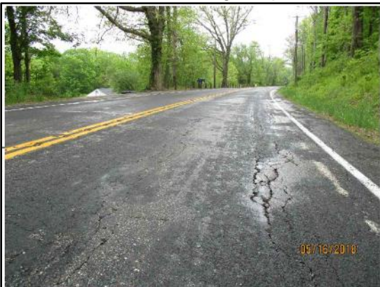
EXISTING: PAVEMENT SURFACE CONDITION
