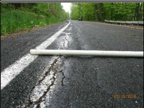
EXISTING: PAVEMENT SURFACE CONDITION
