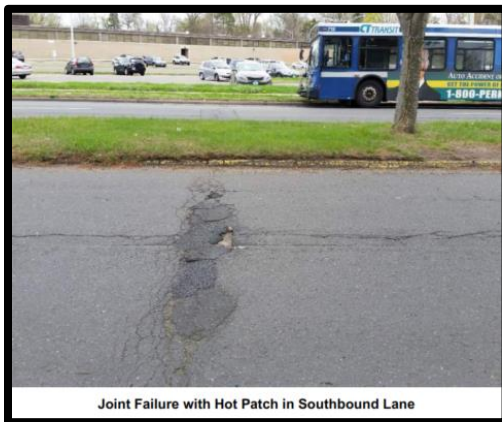
Joint Failure with Hot Patch in Southbound Lane
