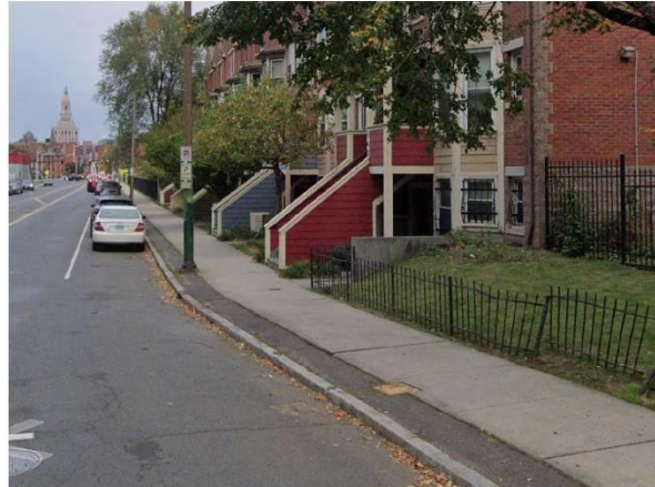
Franklin Avenue has sidewalks in good condition on both sides of the corridor
