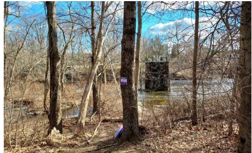
Exhibit 3-1: Abandoned rail abutment north of Tariffville Park crossing north towards Route 189 (Exhibit 3-3, Location B)
