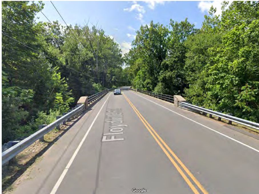
Exhibit 4-12: Existing Floydville Road bridge across the Salmon Brook (Source: Google Maps Streetview)
