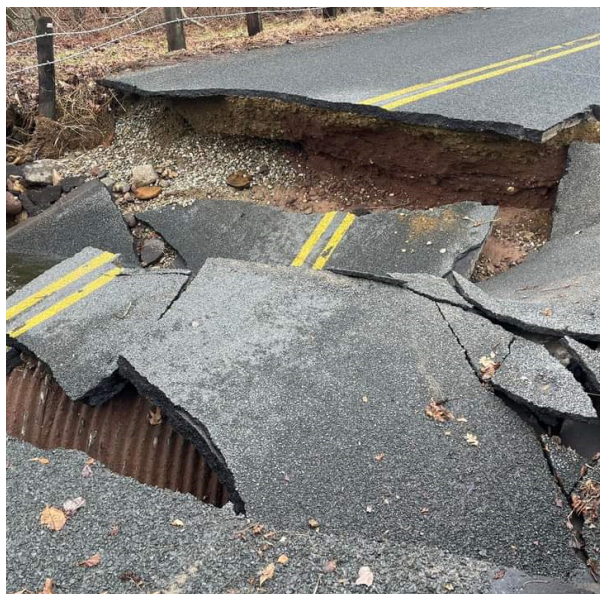
Figure 5: Storm damage in January 2024.
