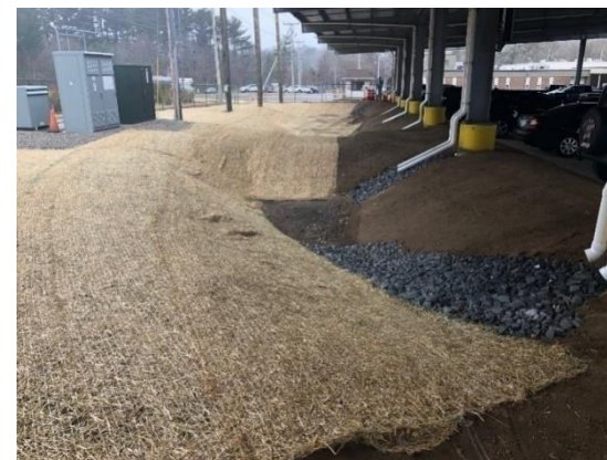
Infiltration basin at an Eversource Facility in Plymouth, MA. Designed by Weston & Sampson
