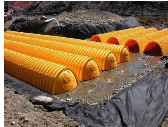
Subsurface infiltration structure, Town of Weston DPW. Designed by Weston & Sampson
