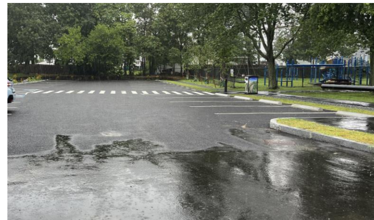
Porous pavement parking in Lynn, Massachusetts. Designed by Weston & Sampson
