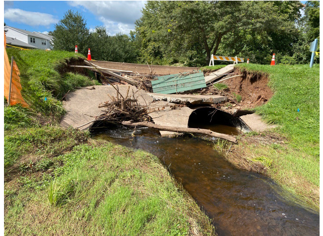
Summer 2021 Damage; Photo Courtesy of Town of Manchester
